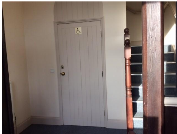
Image of door to accessible toilet 1
